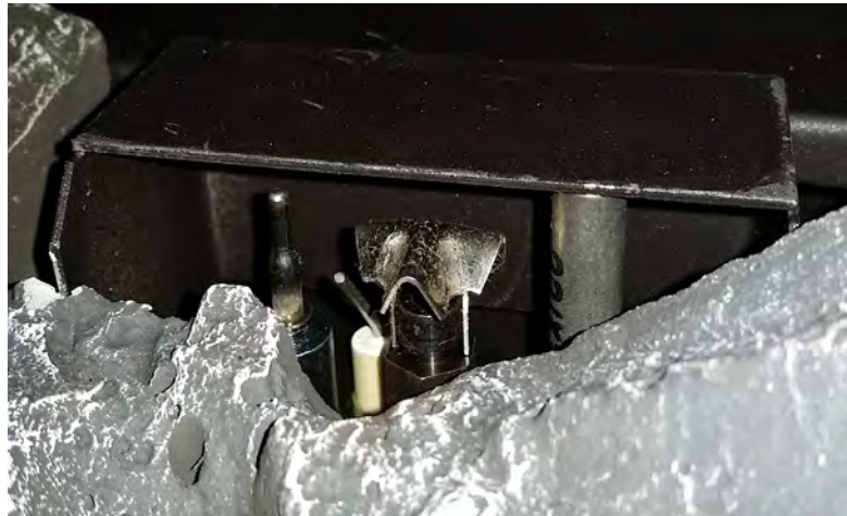
Figure 18. Pilot assembly beside the burner.
